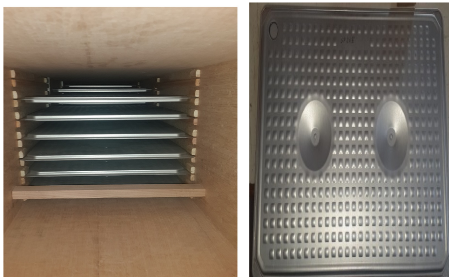
Fig. 4 Installation of PCM in the duct and the shape of PCM Plates.
